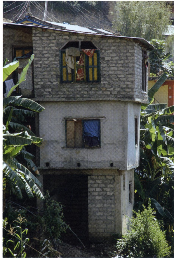
Photo 3: Partly framed Reinforced Concrete with soft storey and vertical irregularity (unsupported columns on upper floors) (Photo: J. ANHORN 2012)
